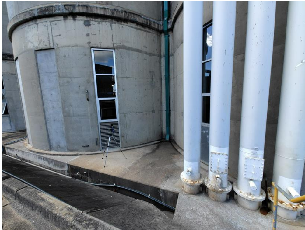
Figure 6.2: Noise Measurement at Blower Louvres
